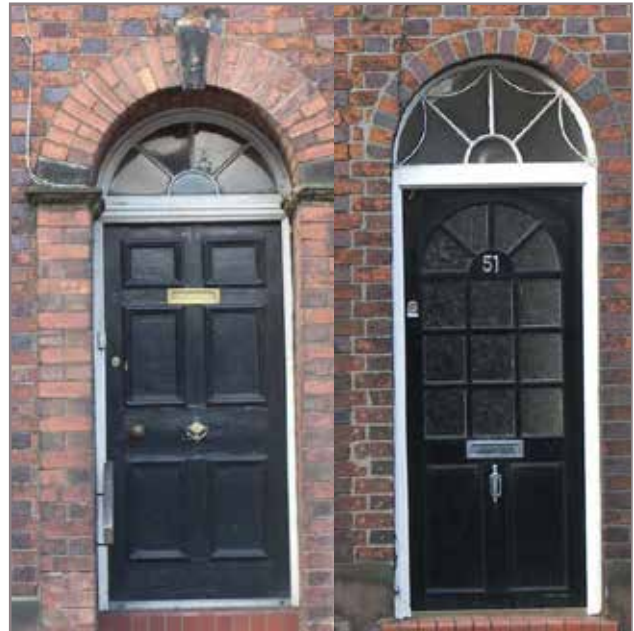
6.17 The use and misuse of fanlights a) over a traditional door b) over a crude pastiche of itself
