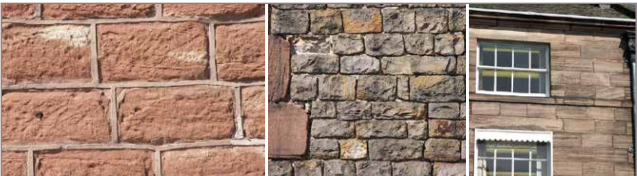
6.4 Stone: a) Inappropriate strap pointing b) Contrasting qualities of stonework on 2-4 Church Street c) Finely detailed ashlar at Ford House.
