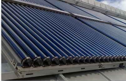
Example of Solar Thermal unit
