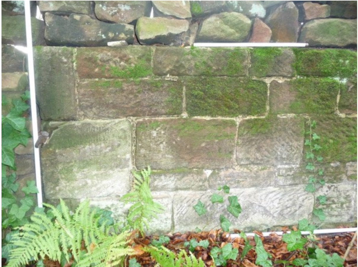
photograph A.4b Photograph A.4b shows a close up of a section of the original stable block building with finely tooled, dressed ashlar courses bonded in their original positions
